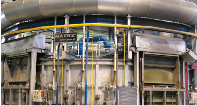
Rotary table furnace
