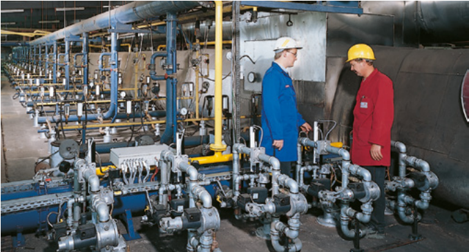
Gas train in a brickworks
