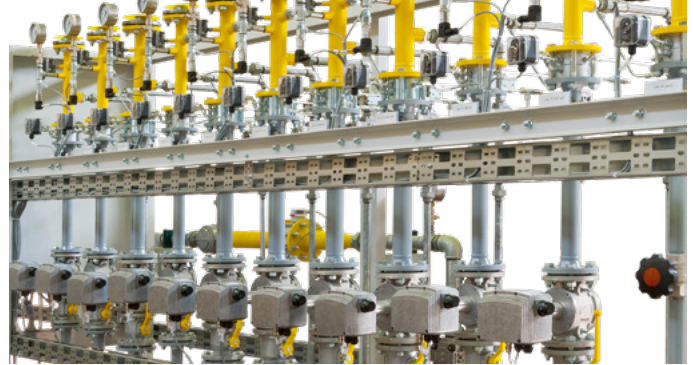
Mixing system in the glass industry
